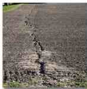
1.2 Erosion - Formen - Rillen Mar 3, 2009 photos: 27
